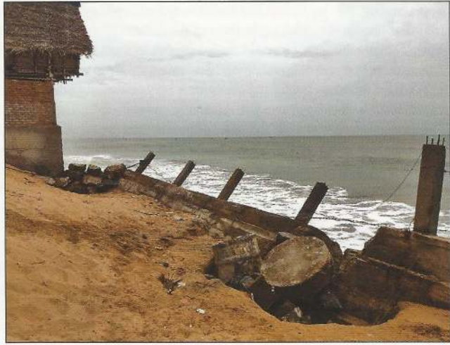
The undermined concrete wall at Repos
