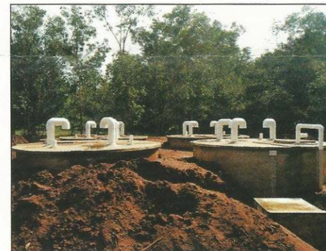
Water tanks for the City Area
